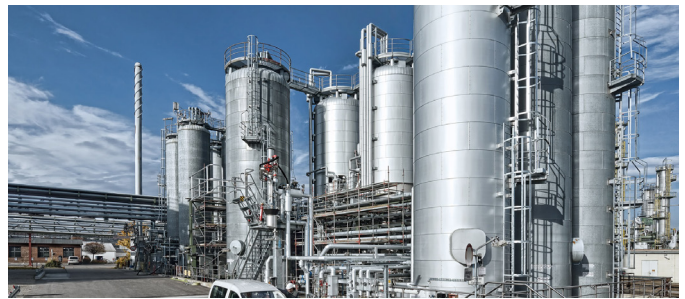
InfraServ Gendorf operates GENDORF chemical park - the largest of its kind in Bavaria, while also providing integrated solutions for core processes operated by companies in the chemical and process industry.
